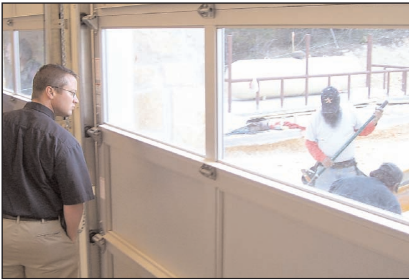
Fire Chief Shawn Wherry keeps an eye on construction at Station No. 5, which is scheduled to open this summer.
